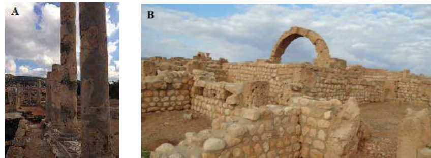
Figure 5. A) Concrete restoration of columns; B) Bad building restoration both in Apollonia City.
